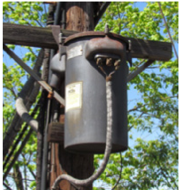
Electrical transformers manufactured prior to 1977 may still contain PCBs. (Photo: Wikipedia)
